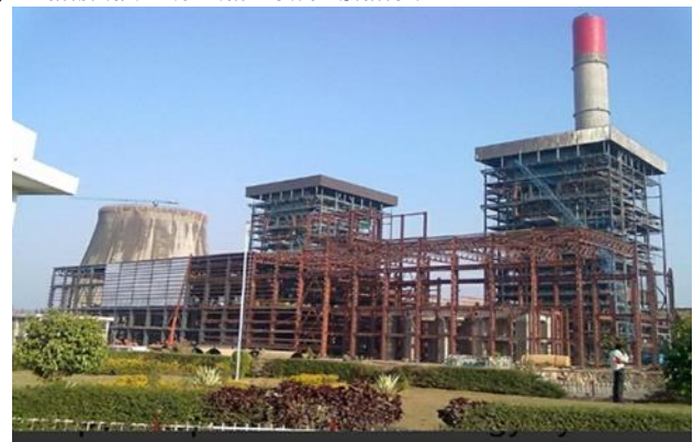
Fig. 6. Kalisindh Thermal Power Station
