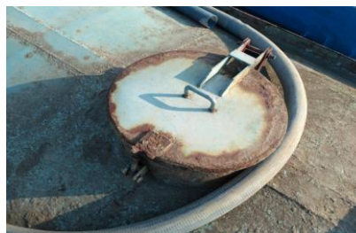
Fig. 4. Corrosion on cap of the pouring valve
