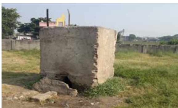
Fig. 4(b). Water /Air towers
