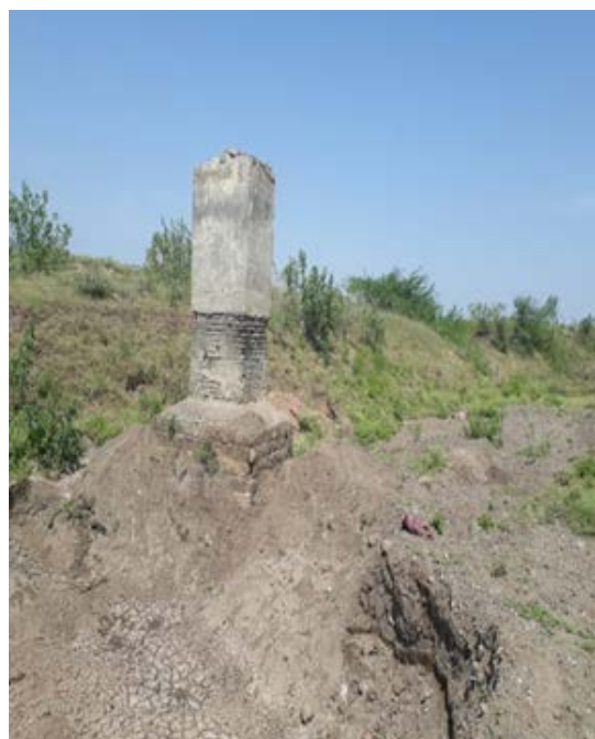
Fig. 4(a). Water /Air towers
