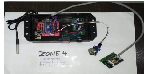
Fig. 8. Boundary monitoring unit
