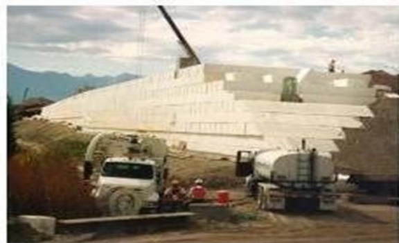
Fig. 2. Typical geofoam embankment construction on the I-15 reconstruction project in Salt Lake City
