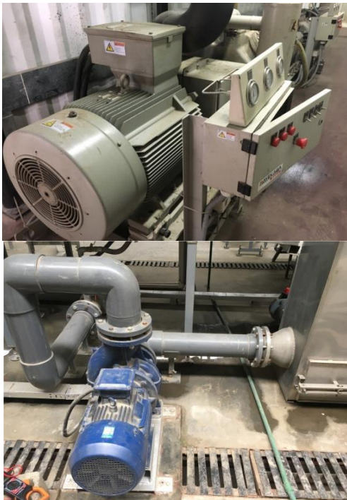
Fig. 4. View of Compressor units of Himfresh Agro Produce Pvt. Ltd. Cold Store Plant
