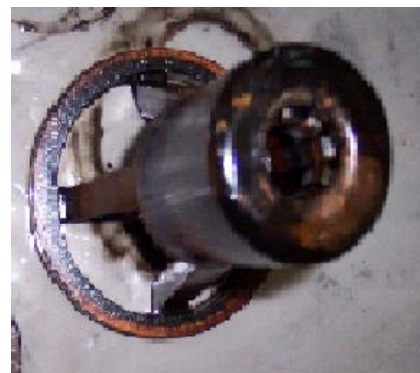
Fig. 1. Contact failure example
