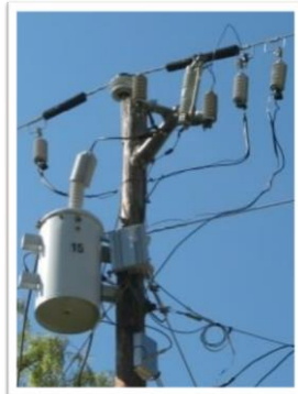
Fig. 3. Repeater connected to the electric pole
