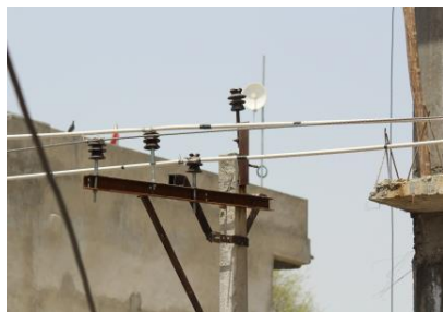
Fig. 2. Power line at Ramganjmandi is covered up with plastic coated tubes to prevent electrocution
