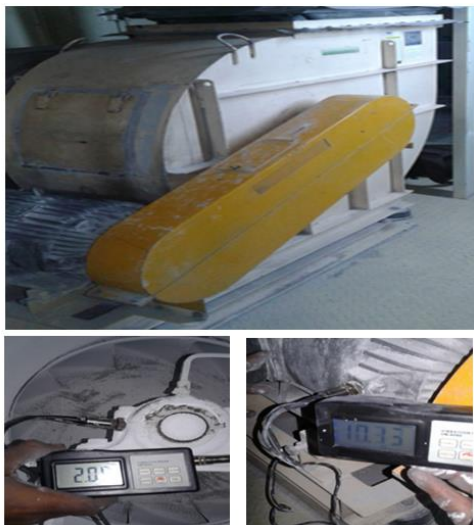
Fig. 2. The vibration data retrieval position
