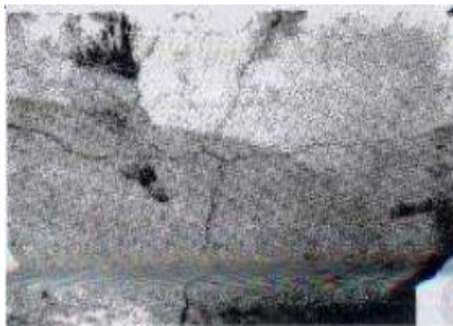
Fig. 3. Drying shrinkage crack
