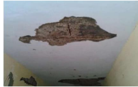
Fig. 5. Steel corrosion induced cracking
