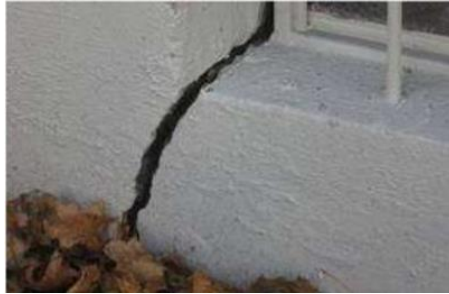
Fig. 2. Plastic settlement cracking
