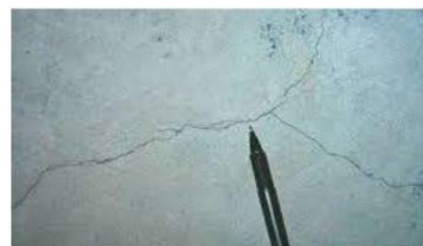
Fig. 1. Plastic shrinkage crack
