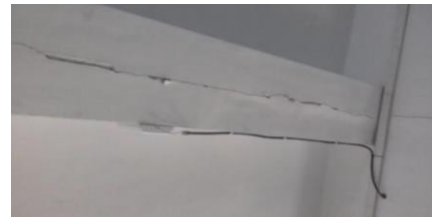
Fig. 9. Damaged expansion joint
